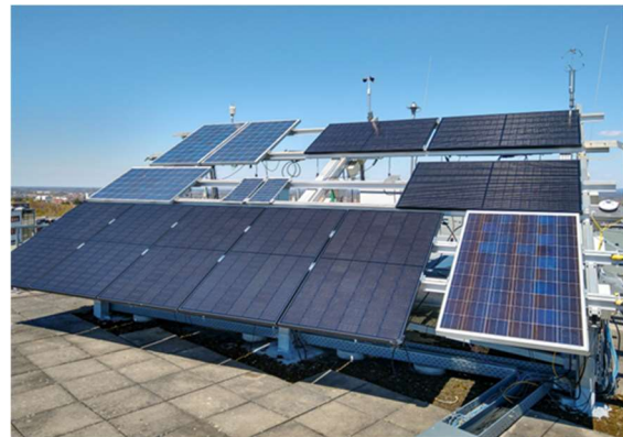
Figure 6: Configuration of PV modules of PV outdoor laboratory for electrical energy yield comparison of microinverters using eight equal, calibrated PV modules (of 360 W p each) as inputs.
